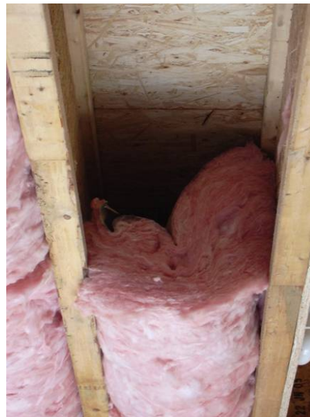
Figure 3.2.2 – Insulation settling away from sub-floor
