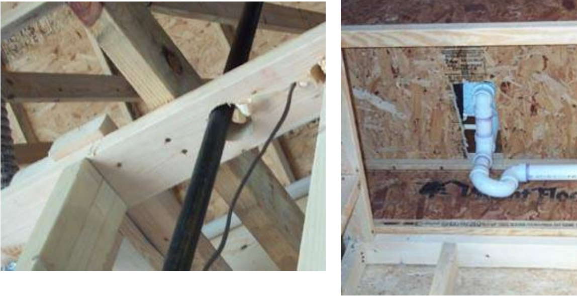
Figure 4.2.1 – Typical piping penetrations leaving large holes
