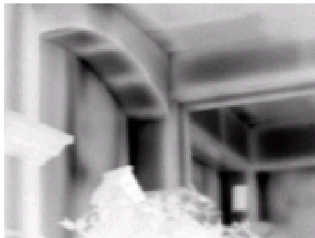
Figure 5.3.2 – Infrared image of dropped ceiling without an air barrier and proper insulation
