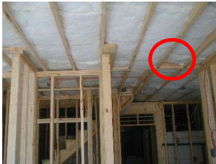
Figure 1.1.6 - Insulation installed with gaps and voids
