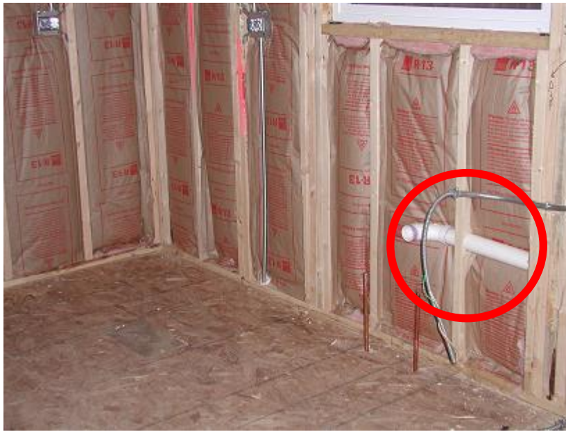
Figure 1.1.5 – Misalignment of insulation due to compression
