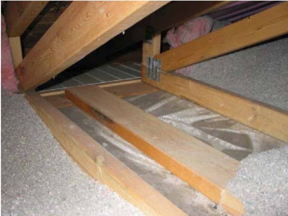
Figure 1.3.1 - Wind intrusion from a soffit vent
