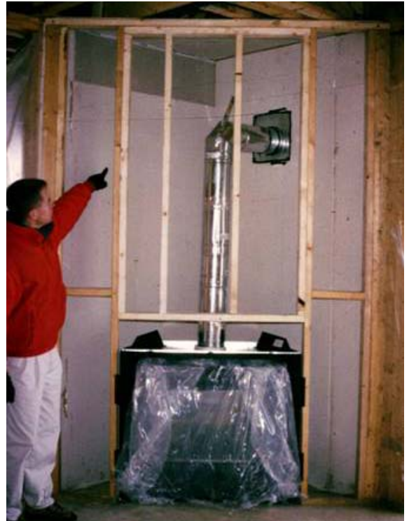
Image courtesy of Building Science Corp
